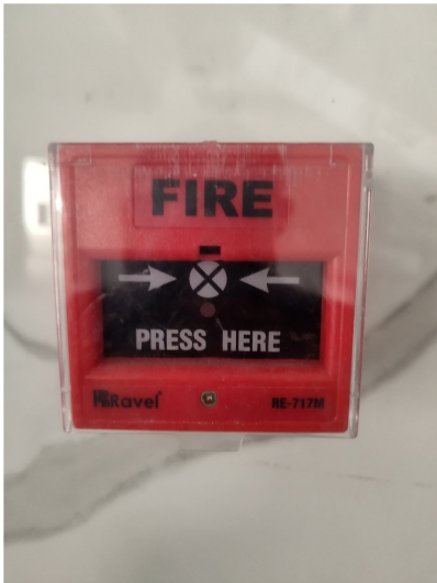
FIRE1057-Fire&Safety-Manual call point-Addressable-No's
