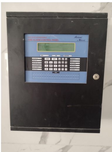
FIRE3509-Fire&safety -fire alarm panel single loop-No's
