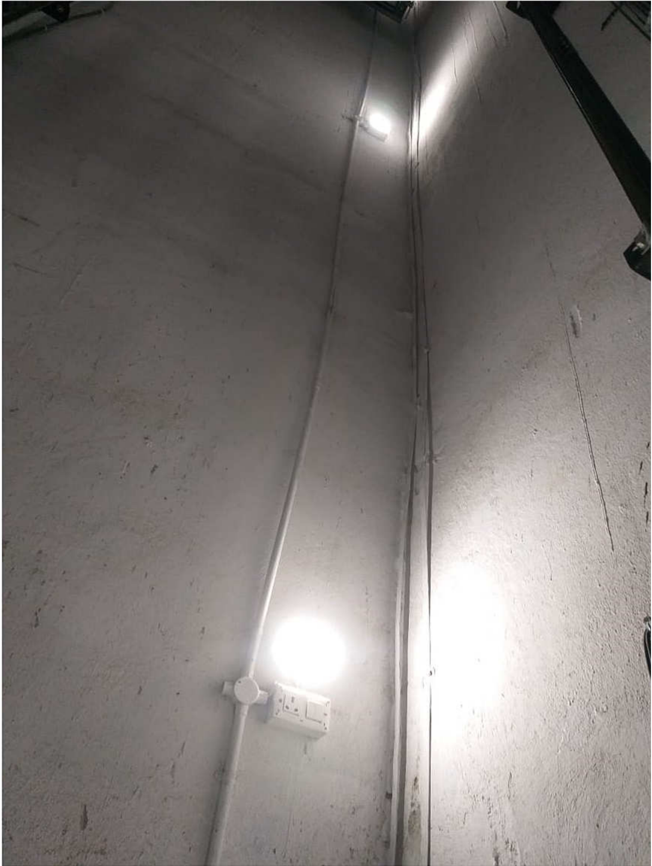
A typical picture showing electrical connection, lighting in lift shaft.
