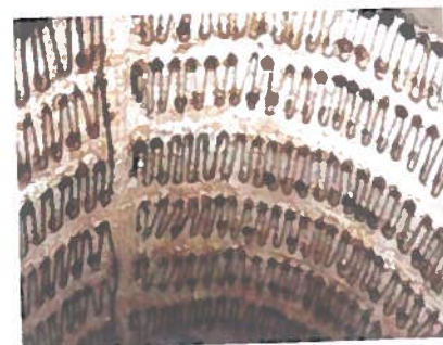
Inside Furnace View
