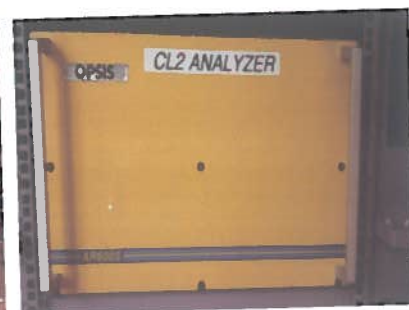
Online Chlorine gas Analyser
