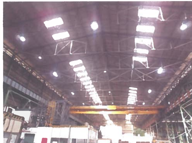
LED lights mounted in the bay
