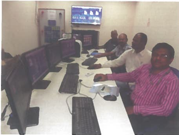
Central Control Room – Utilities, NFC
