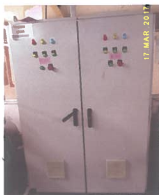
Control Panel installed on C & D Head machines
