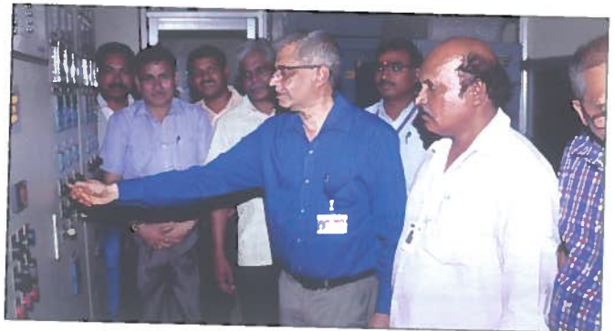
Shri G. Kalyanakrishnan, Chairman & CE, NFC switching on the Board to inaugurate sintering furnace at CFFP-P.
