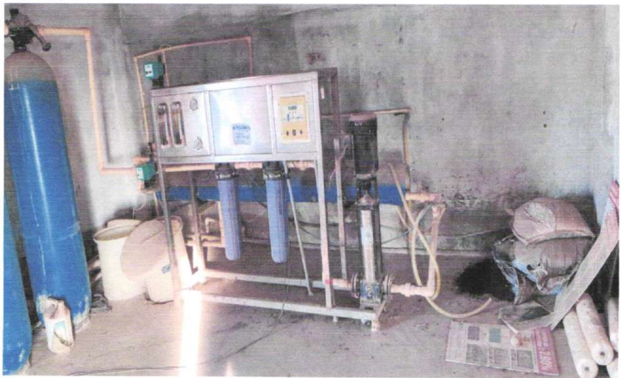
WATER TREATMENT PLANT NOT WORKING
