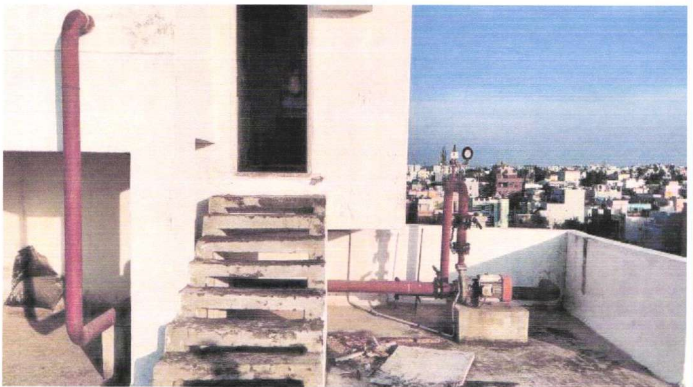
TERRACE FIRE WATER TANK-FIRE BOOSTER PUMP WITH ACCESSORIES
