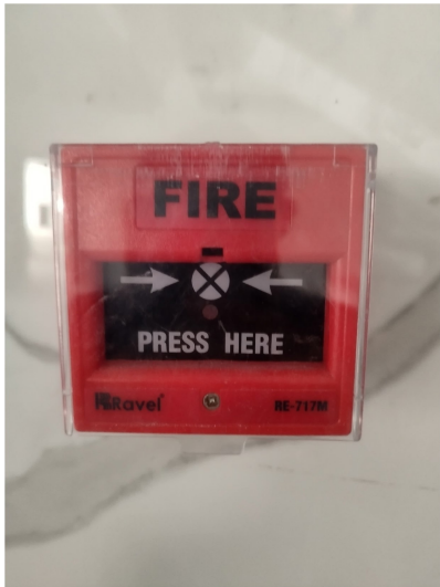
FIRE1057-Fire&Safety-Manual call point-Addressable-No's
