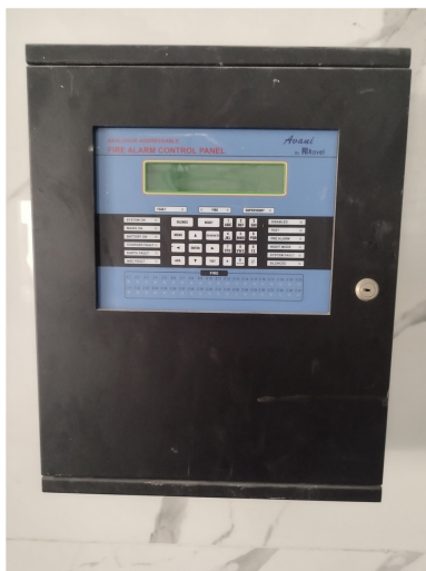
FIRE3509-Fire&safety -fire alarm panel single loop-No's
