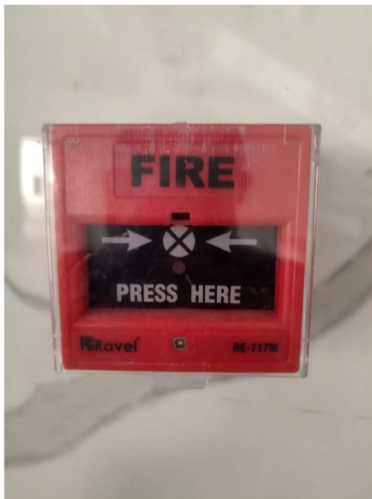
FIRE1057-Fire&Safety-Manual call point-Addressable-No's
