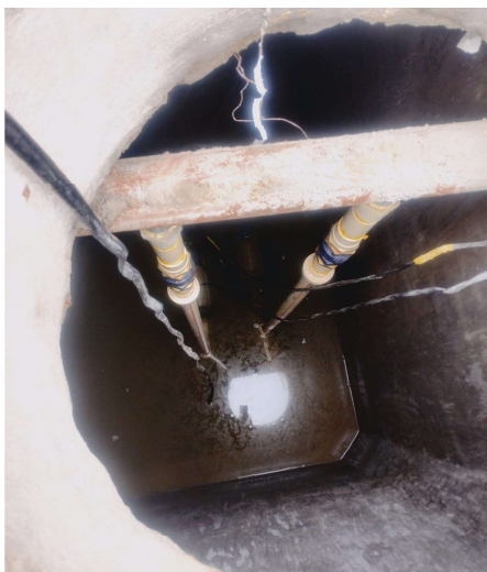
PLUM1531- Plumbing -Horizontal open
