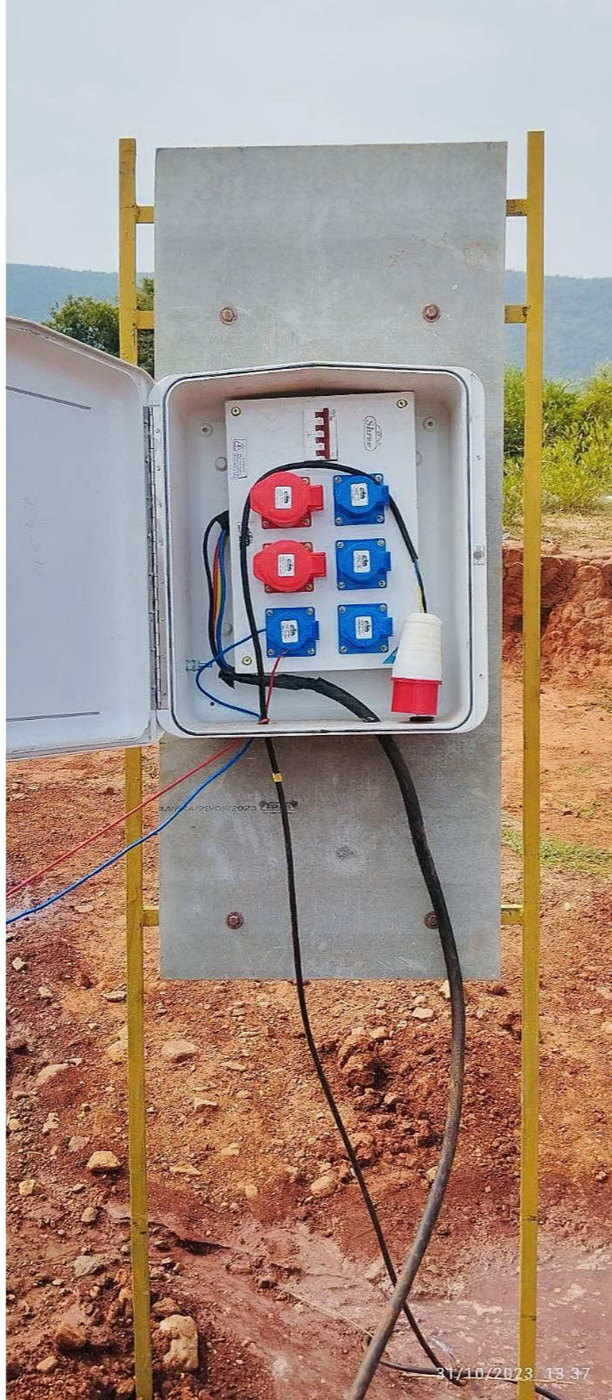
ATypical Picture Showing MS Stand with Industrial DB Box As Installed
