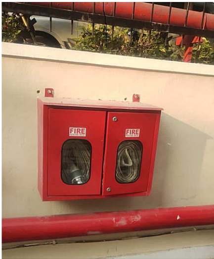
FIRE1291-Fire & Safety-Hose Box-Double Door-Nos
