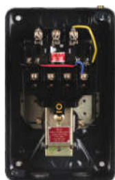
Interior View of MK1 DOL
