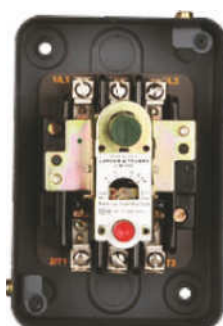
Interior View of MF1 DOL - 3Ø Starter
