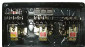
Interior View of MK1 SASD
