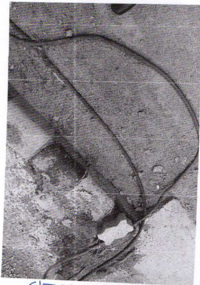
Street light wored not loose kept on ground
