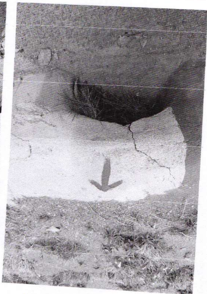
Storm water Humapores damaged.
