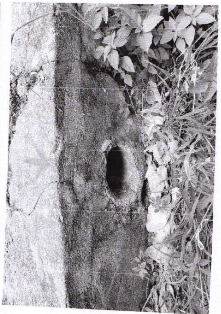
Home pipe damaged
