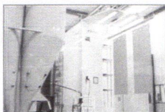
Fully automated paint finish unit
