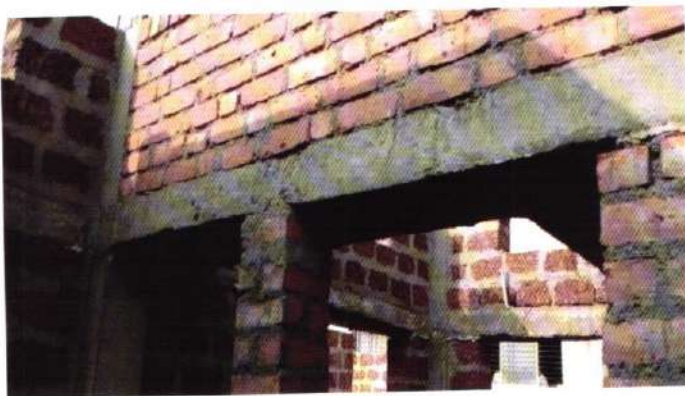
uneven surface need to chipping work
