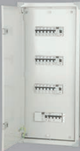
Vertical Per Phase Isolation Double Door DB
