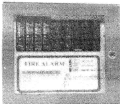
Fire Alarm Control Panel
