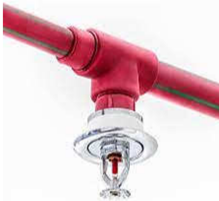
FIRE6625-Fire & Safety-Fire fighting-Fire sprinklers-No's
