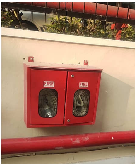
FIRE1291-Fire & Safety-Hose Box-Double Door-Nos
