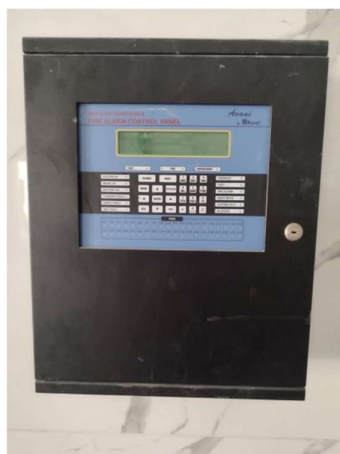
FIRE3509-Fire&safety -fire alarm panel single loop-No's
