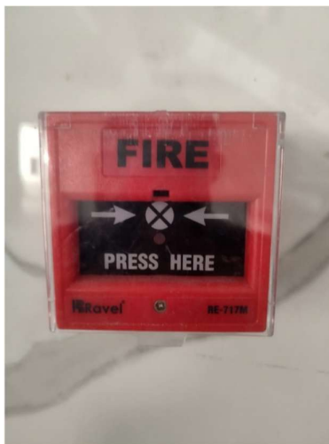
FIRE1057-Fire&Safety-Manual call point-Addressable-No's
