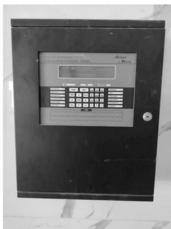
FIRE3509-Fire&safety -fire alarm panel single loop-No's
