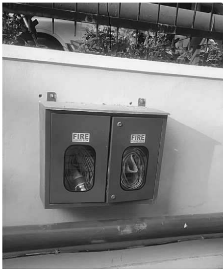
FIRE1291-Fire & Safety-Hose Box-Double Door-Nos
