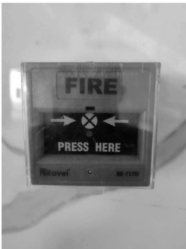
FIRE1057-Fire&Safety-Manual call point-Addressable-No's
