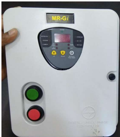
ELEC4446-Electrical-DOL Automatic Starter-Single phase -with dry run protection -L&T-MR-Gi- CS91322NCOG-Nos
